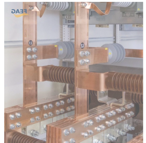
LV Switchgear type ZR-V Internal protection degree - Color RAL - 7035 Rated current of main bus - Rated voltage - 400V
